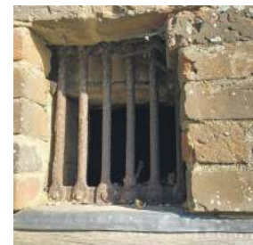
Grill window Docking lock up
